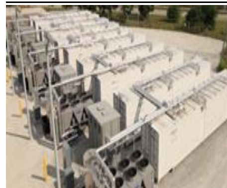
Figure 76: AES 100MW Li-ion battery plant
